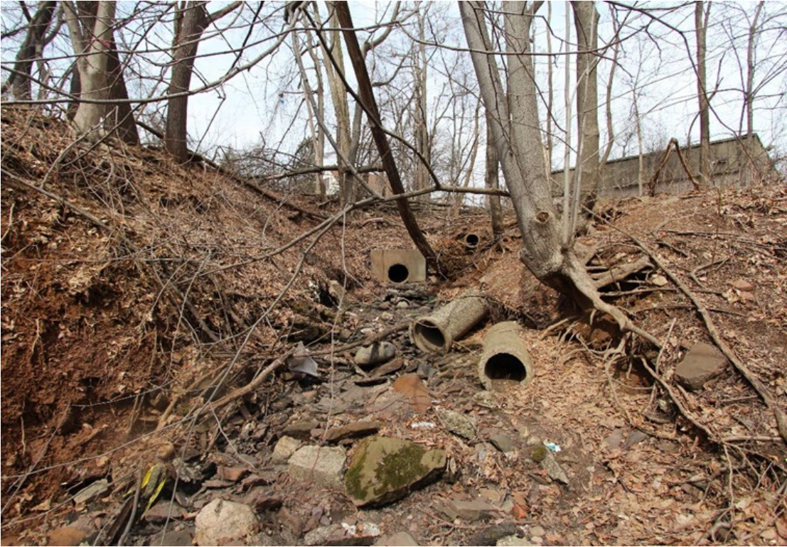
Stormwater Canyon Before
