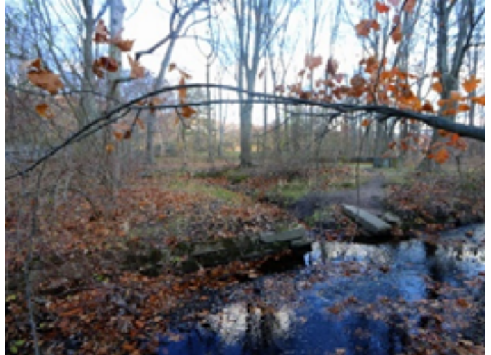
Figure 9. Incised stream channel at Van Saun Park is disconnected from the floodplain, creating conditions that lead to degradation and destabilization downstream (Courtesy of Biohabitats).
